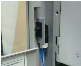
Door Switch in Access Level 1
