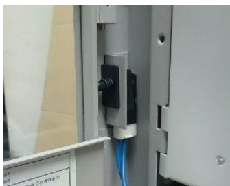
Door Switch in Access Level 1
