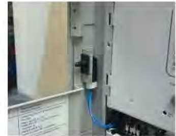
Door Switch in Access Level 2
