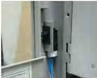
Door Switch in Access Level 1
