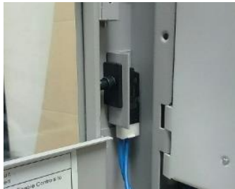
Door Switch in Access Level 1
