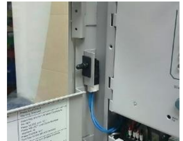
Door Switch in Access Level 2
