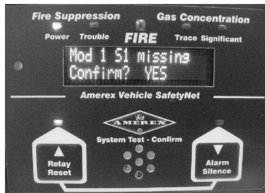
Figure 7 - Missing Sensor Confirmed
