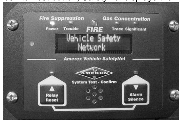
Figure 9 - System Test Button Pressed
