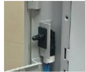
Door Switch in Access Level 2
