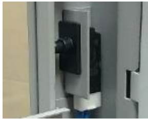
Door Switch in Access Level 1
